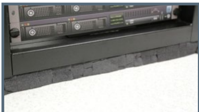
Above, below and between racks
