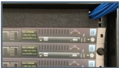
Blanking inside racks
