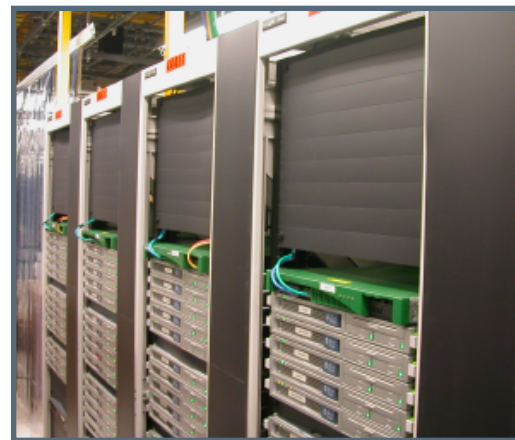
Fill Gaps Between Racks
